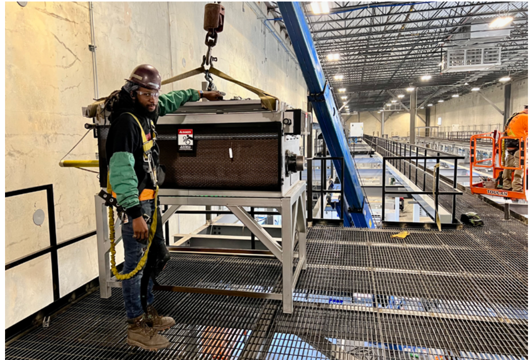
Millwright team rigging 3,000 lb motors for elevated conveyor line at a new UPS regional hub
